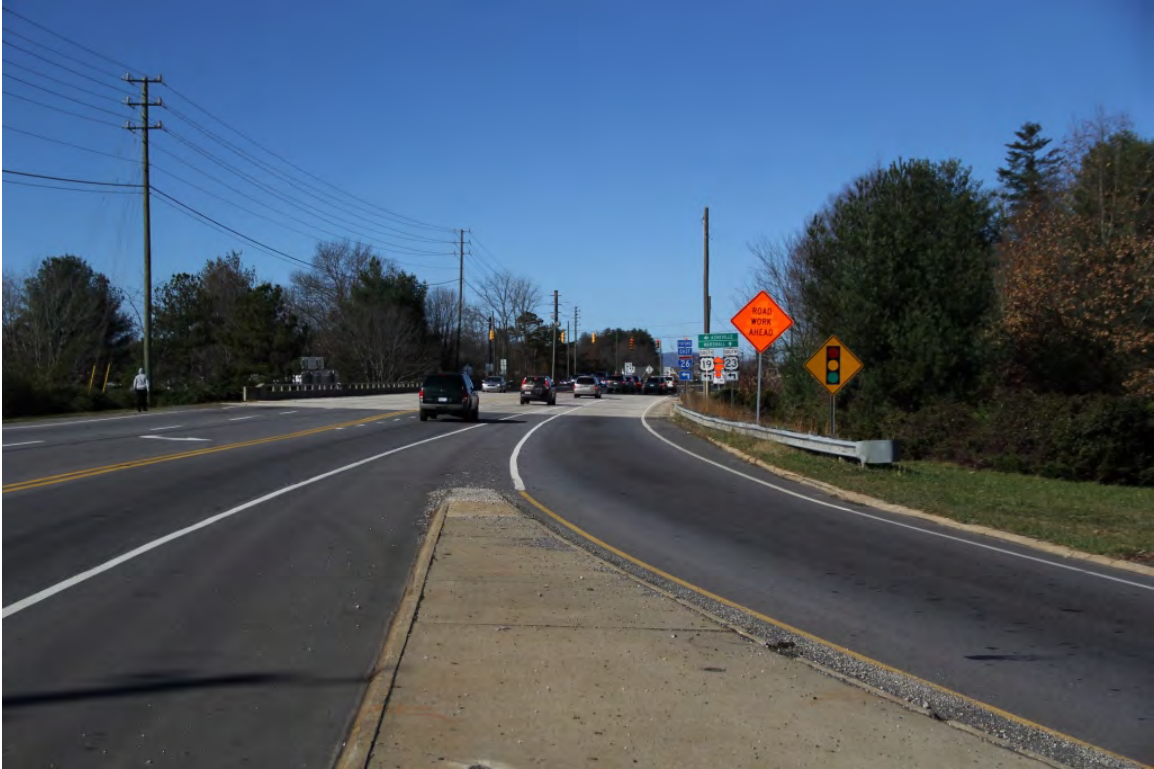
Bridge No. 382 on US 25-70 (Weaver Boulevard) over US 19-23, Exit 19, view to west
