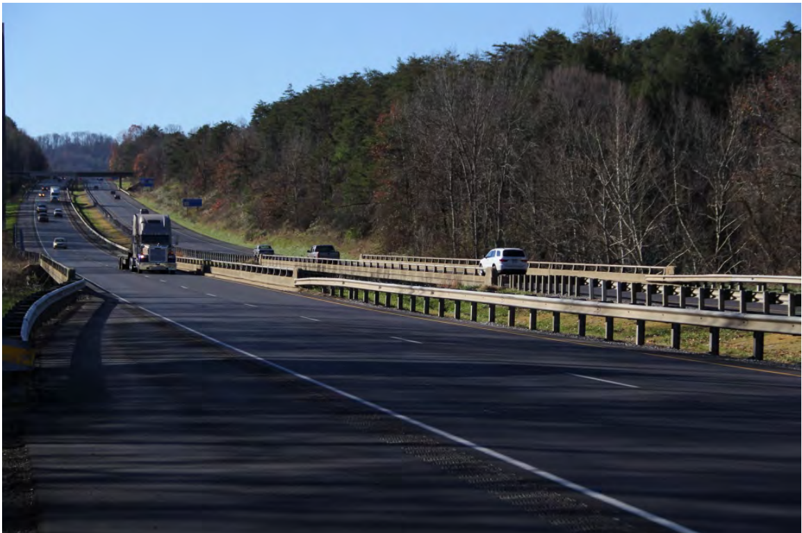
Bridge Nos. 370 (l) and 373 (r) on US 19-23 over Reems Creek, view to southwest
